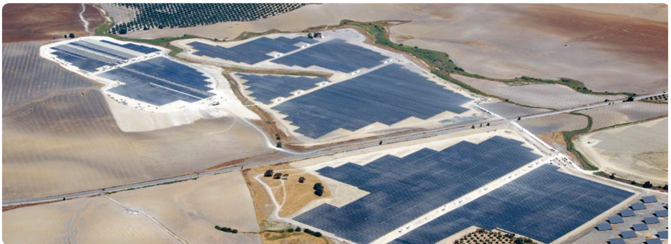
PHOTOVOLTAIC SOLAR FARM, ESPEJO, CÓRDOBA.
